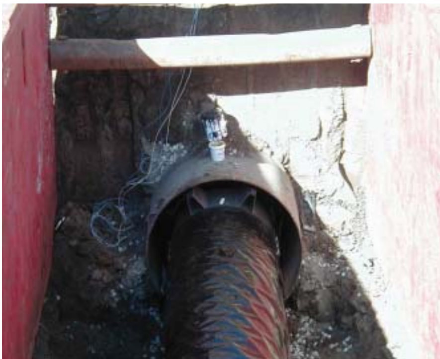
Electrical isolation in casing sleeve at road crossing.
