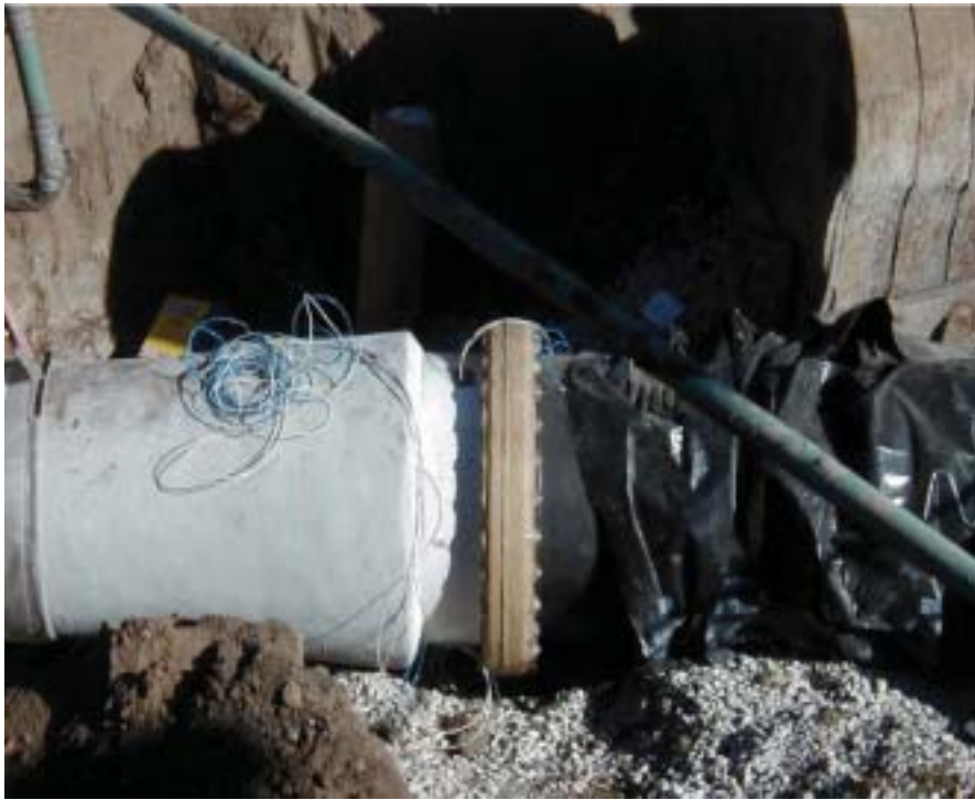
Flange isolation at tie-in to existing water main.
